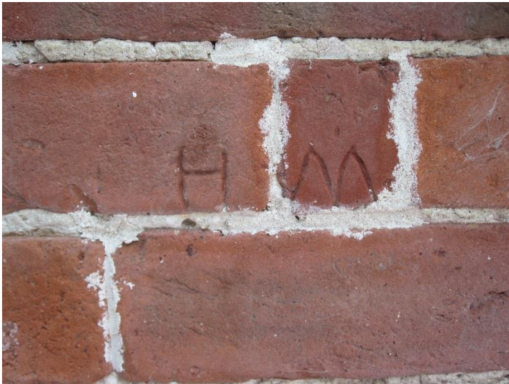
Harold Mead's initials can be seen today scratched in a wall at Court Lane Farm
